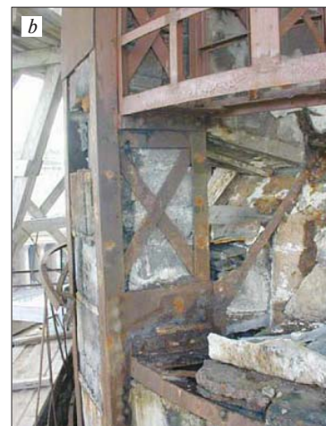
Fig. 9. Upper (a) and lower (b) parts of the metal frame of the dome
